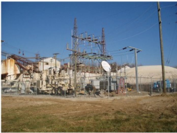
Hughes powers SCADA connectivity for electrical substations
