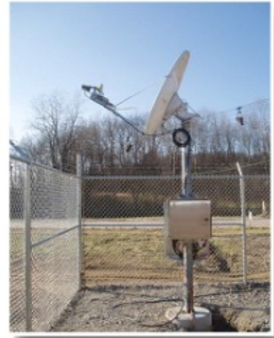
Hughes SCADA solution include option for outdoor enclosure
